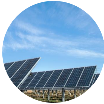
Considering PPA Solar
