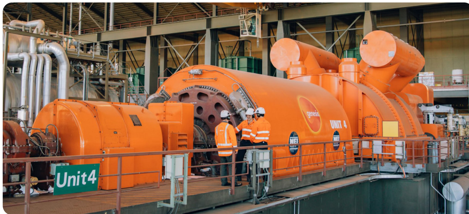
The Rankine hall at Huntly Power Station.
