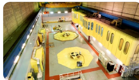
📍 The turbine hall in the underground Rangipo Power Station
