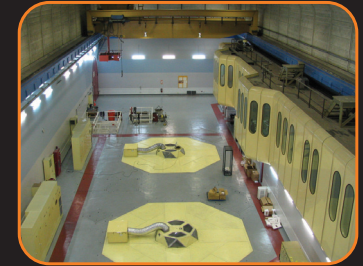
RANGIPO POWER STATION (120 MW) [underground]
